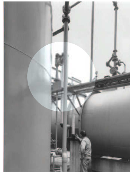
Stock Fig. 7014 scrubber system, used to remove HCL fumes during tank venting, illustrates the benefits of a compact lightweight system.
